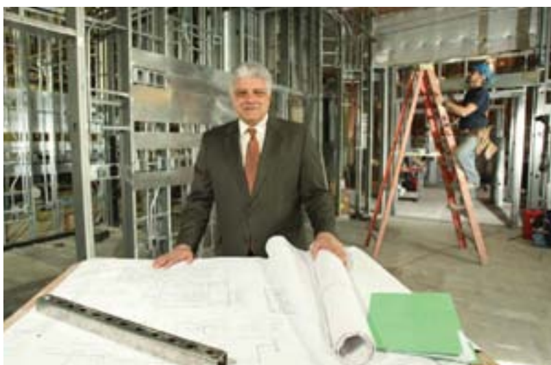
Frank J. Vozos, M.D., FACS, president and chief executive officer of Monmouth Medical Center, a surgeon who trained and practiced at Monmouth, is shown above in an OR construction area.
